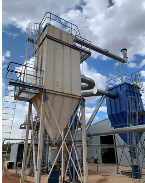
Image 5. DP6 - EBF Baghouse
